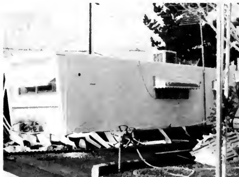
Photo 10. Mobile home shifted off its foundations; note damage to skirt. Drew P. Lawrence photo.
